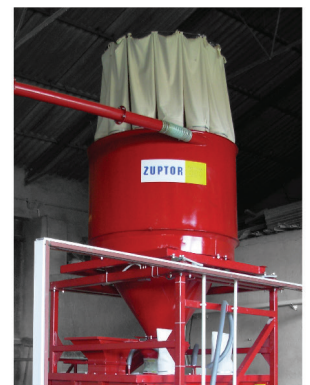
Cyclone tank with filtering system
